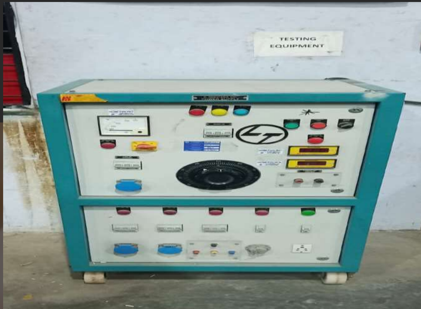
AC / DC TESTING TROLLEY
